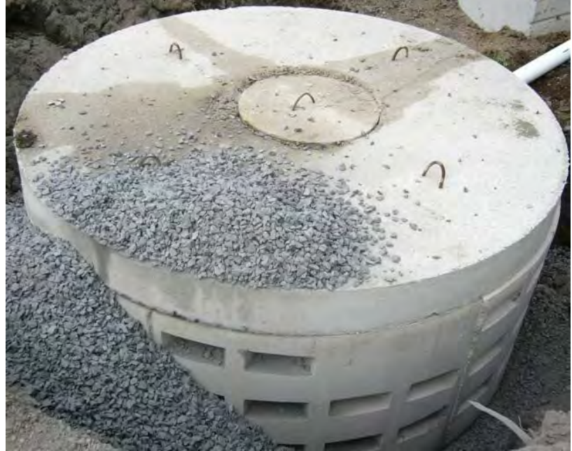
Figure 16: Concrete infiltration well
