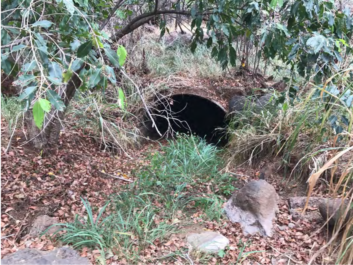
Figure 20: Constriction points like this culvert are already limiting flow of the stream. Retrofitting them with grade controls or stand pipes could increase sediment retention effectiveness.
